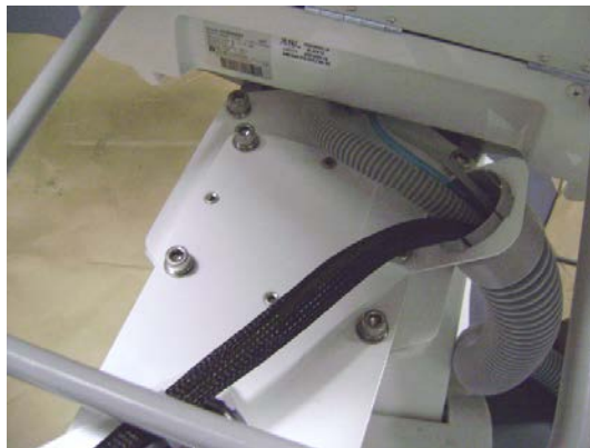
Umbilical from Delivery System is shown installed into Umbilical Duct Hose and routed to J-box. Note: Vac Pac umbilical is also shown routed into Duct Hose in photograph at left.
