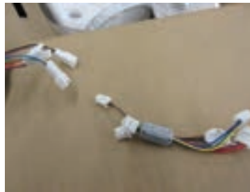
Jumper wire harness with Ferrite is disconnected from light wire harness prior to inserting wire harness through light post and Light Swing Arm Mounting stud. Jumper will be re-connected to the Sensor Switch Box and the umbilical wire harness from the Power Supply Box in a later step
